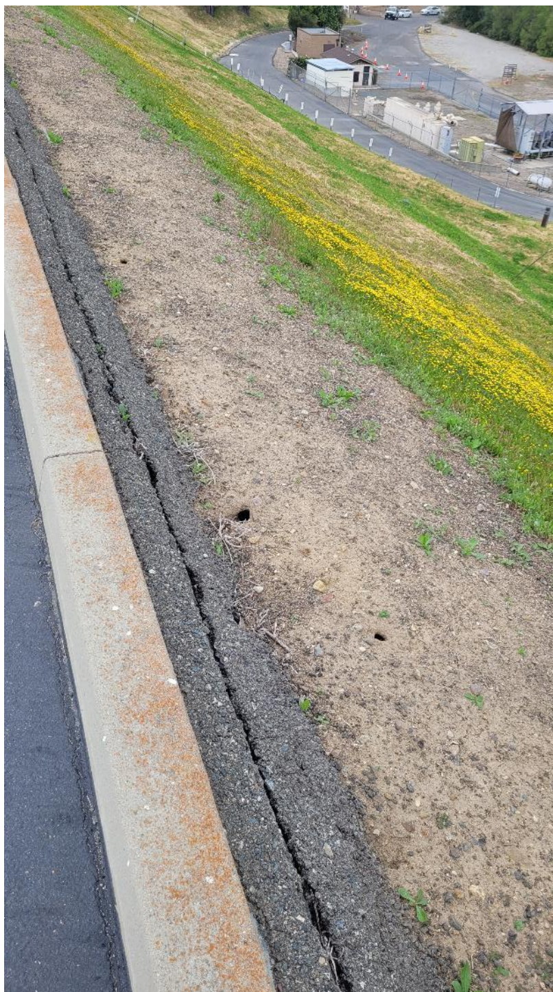
Photo 2: View of rodent holes near the crest and downstream slope.
