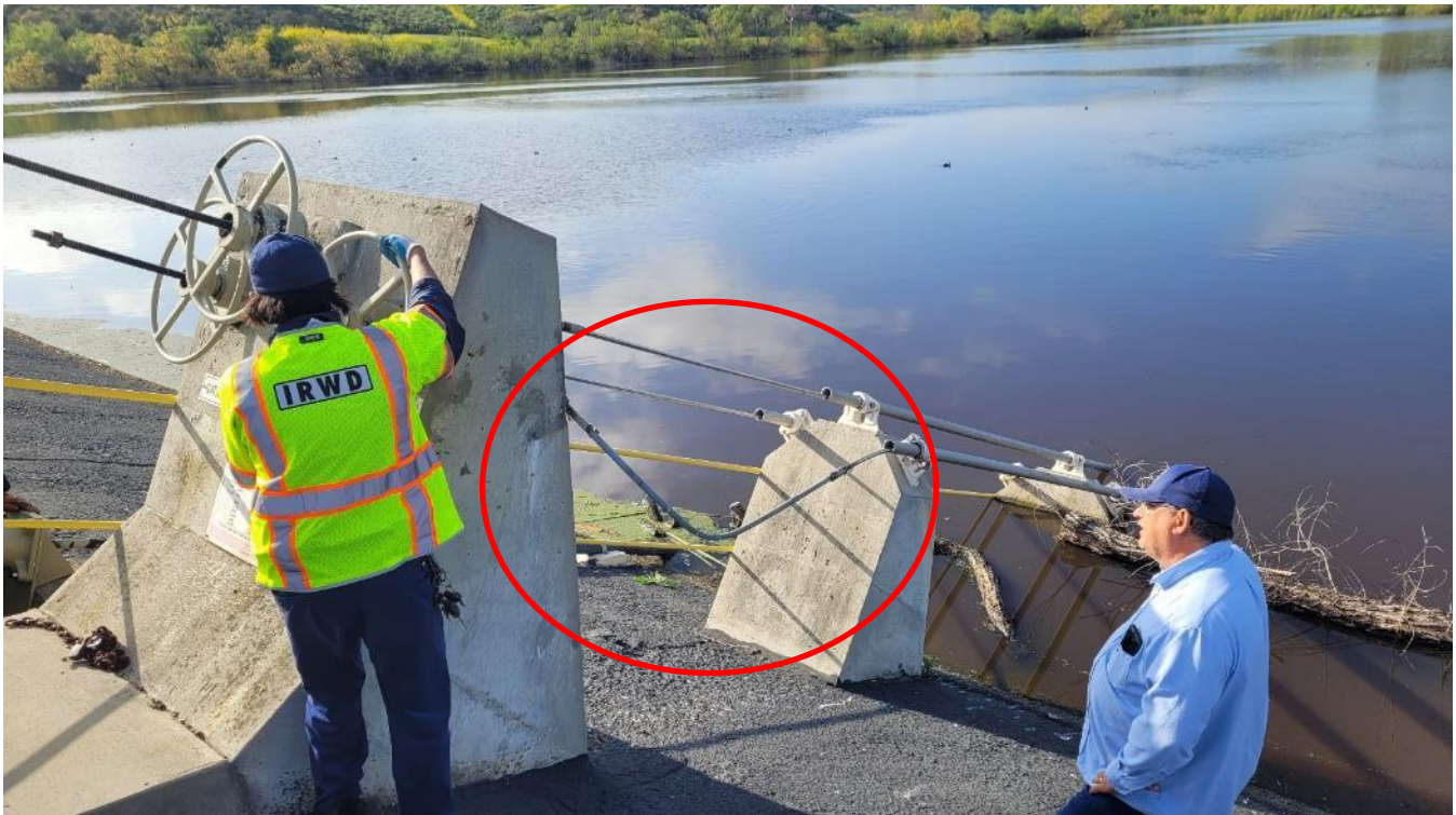
Photo 5: View of the bent slide gate stem.
