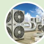
Cooling office buildings
