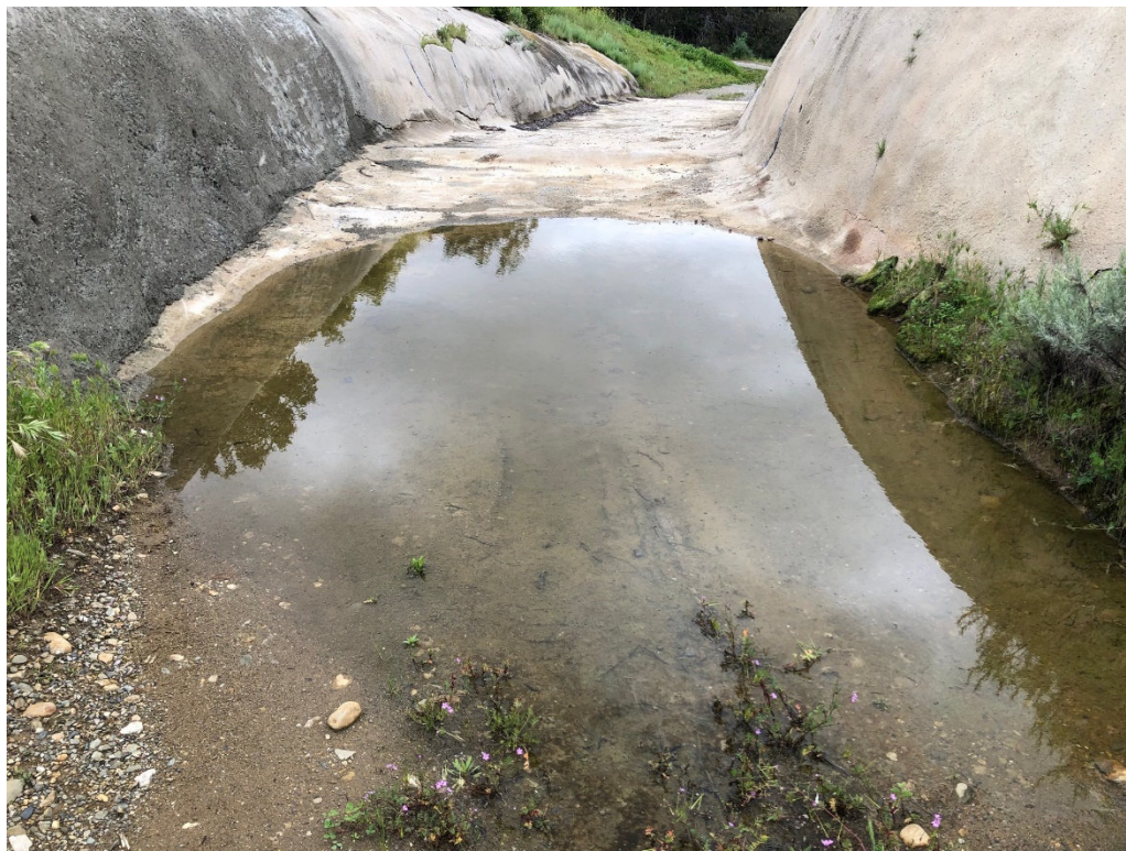
Photo 6: View of puddle in cemented area near southeast corner of the reservoir (facing south).
