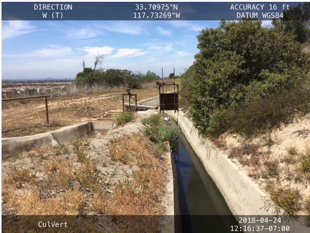
Photograph 10 -Photo west along the abandoned Highland Canal located in the southwest portion of the study area.
