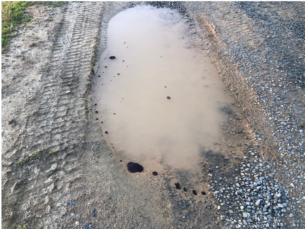
Photo 4: View of puddle on southern access road of reservoir (facing west).
