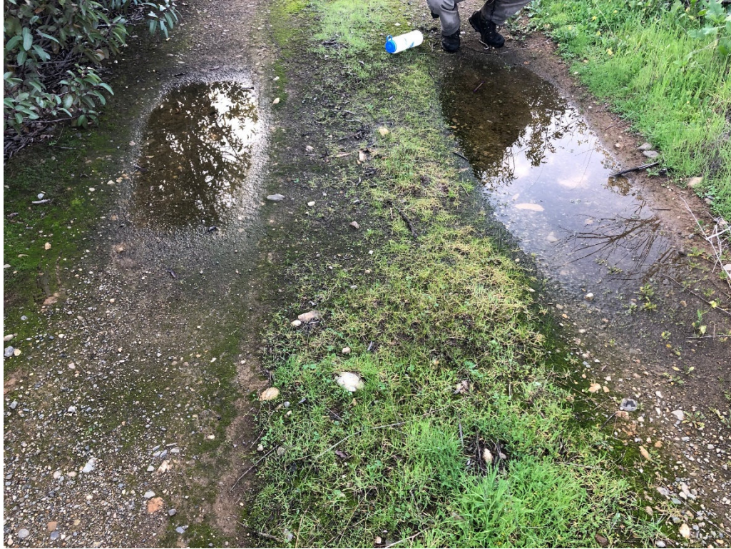
Photo 3: View of road rut puddle in access road on the west side of the reservoir (facing south).
