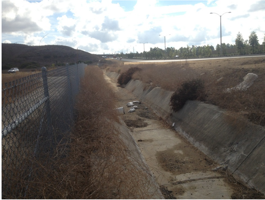
Exhibit E – Photograph is facing south and shows the concrete drainage structure adjacent to Portola Parkway
