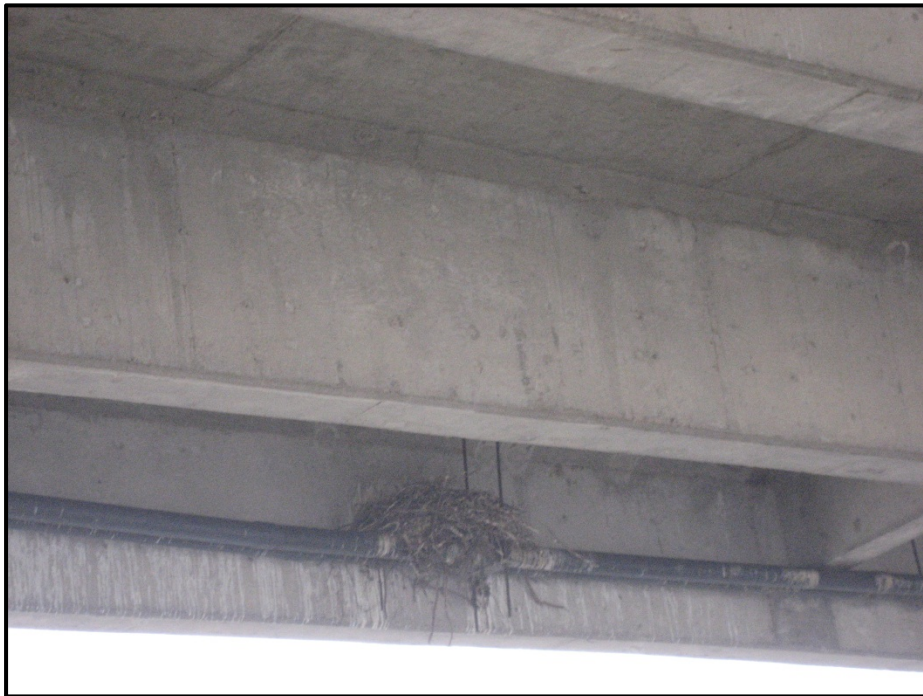
Photograph 2. Photograph depicts an existing stick nest observed during project surveys located on the underside of a bridge crossing Peters Canyon Channel.
