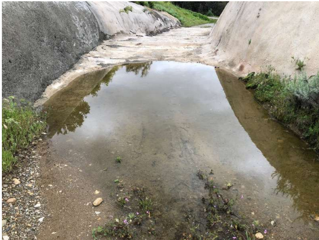
Photo 6: View of puddle in cemented area near southeast corner of the reservoir (facing south).
