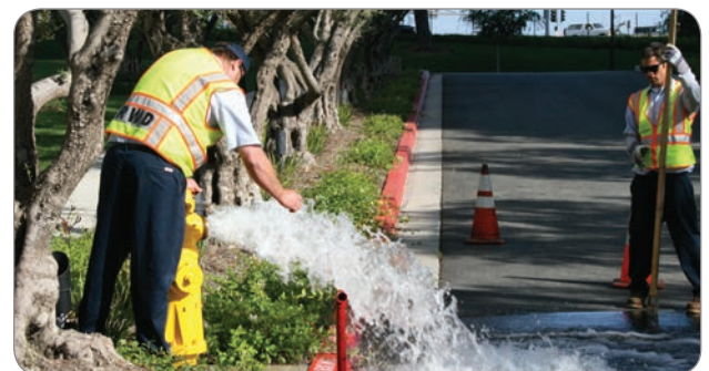
IRWD workers flush fire hydrants to maintain the integrity of the distribution system.
