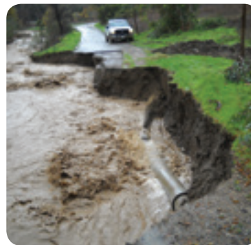
A portion of Williams Canyon Road was washed out, along with 900 feet of a water main during storms and flooding in December 2010.
