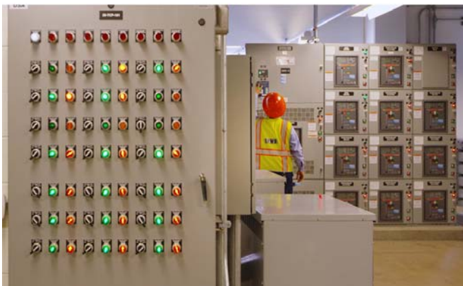
Employee working in Electrical Room
