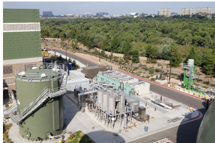
Gas Treatment, Microturbines & Flare
