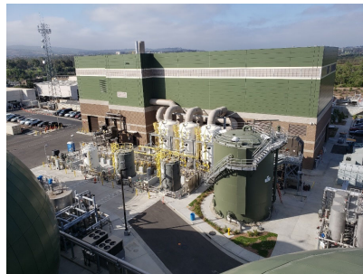
Odor Control System
