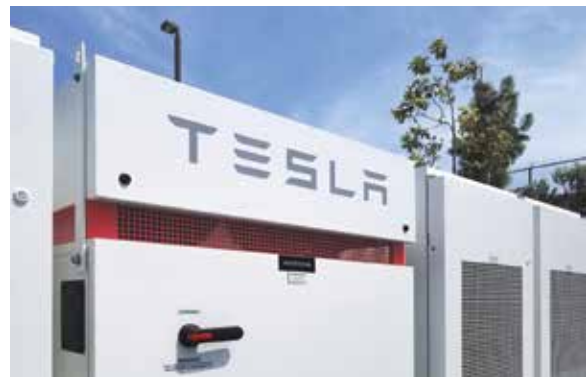
Tesla Battery Station
