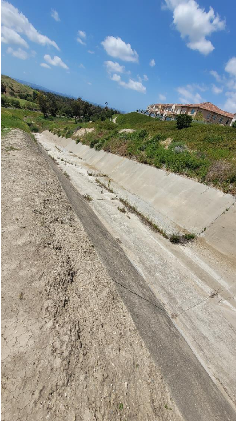
Photo 3: View of the vegetation growth in the cracks and joints of the spillway side channel.
