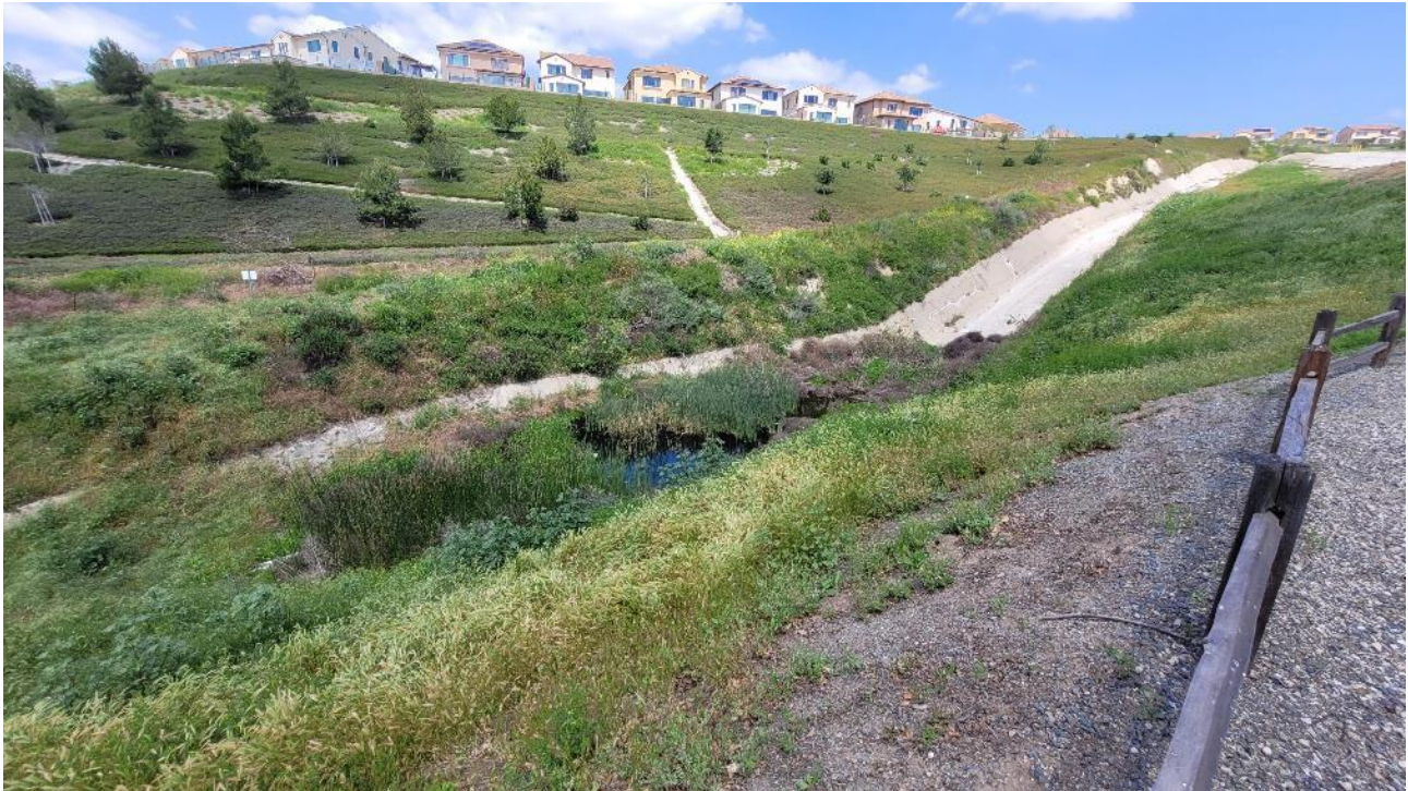
Photo 2: View of the spillway exit with dense vegetation growing within the channel.
