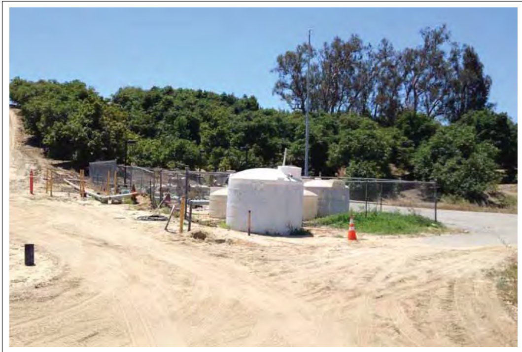
View of disturbed area at the Orchard Hills Facility.
