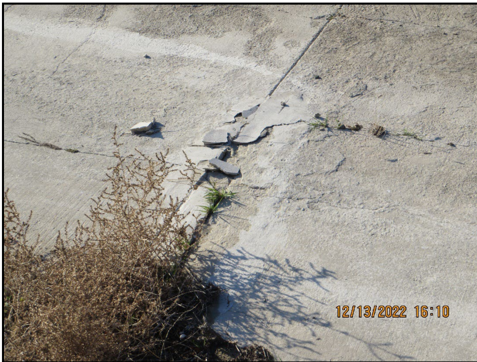
Photo 8) Concrete spalling at previous liner joint repairs.
