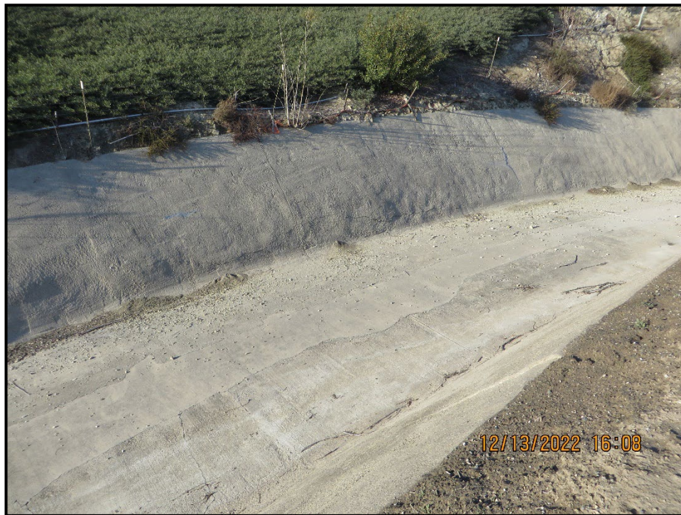
Photo 6) Spillway channel. Note hairline cracking on the right spillway wall and concrete spalling at previous repairs.
