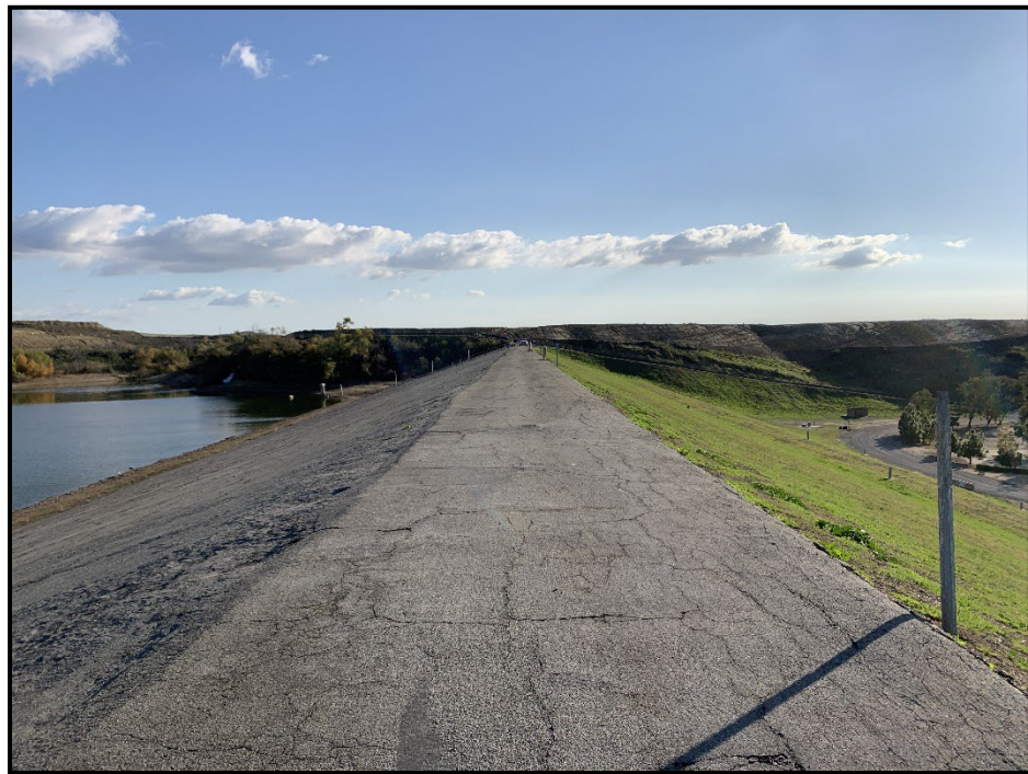
Photo 2) AC-lined crest and upstream face looking towards left abutment. Note cracks.
