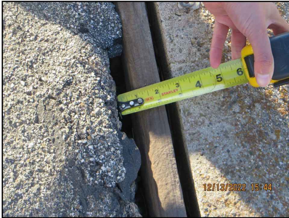
Photo 11) Separation between AC pavement and spillway concrete liner joint.
