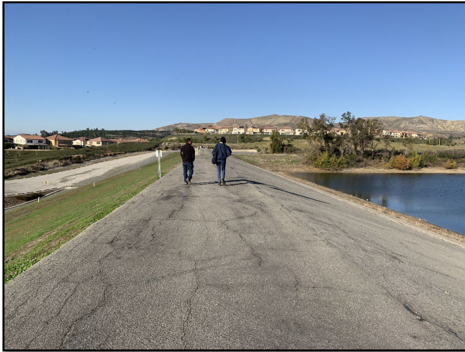
Photo 1 AC-lined crest and upstream face looking towards right abutment. Note cracks.
