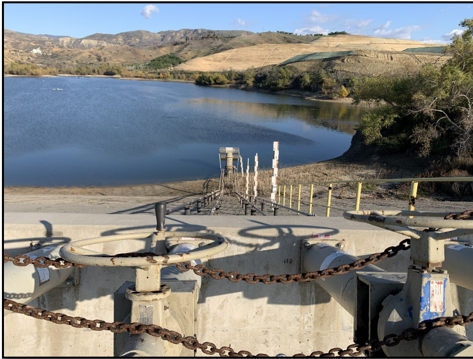
Photo 3) Left end of AC-line upstream face and the reservoir. Note outlet control valves and cleared vegetation near groin.
