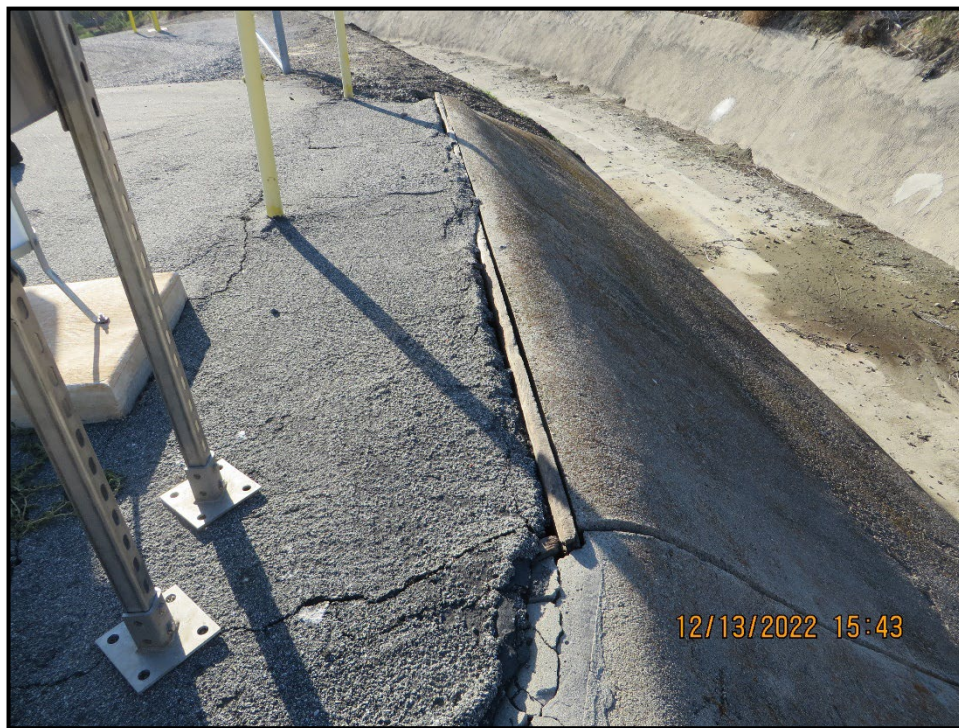
Photo 10) Separation between AC pavement and spillway concrete line joint.
