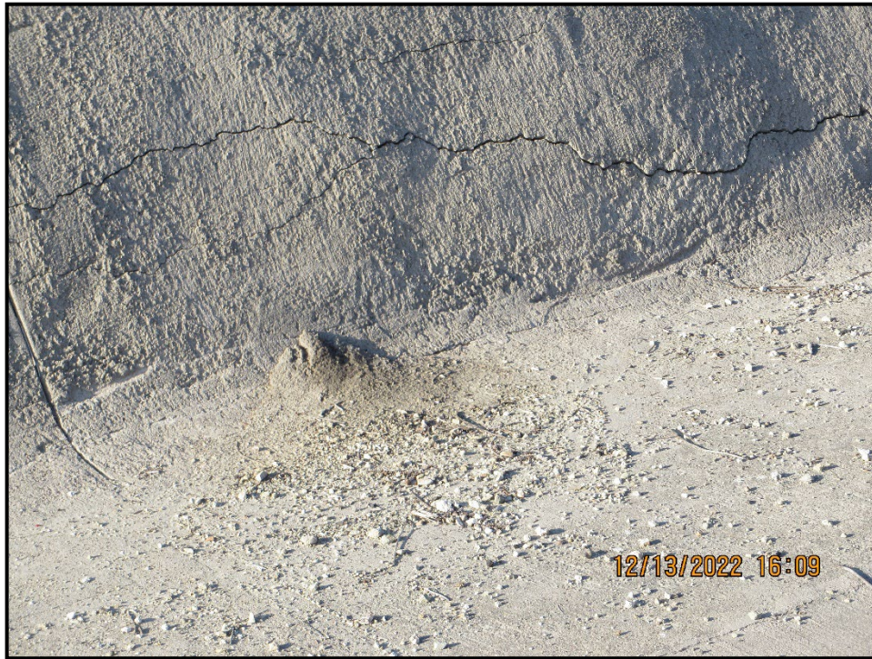
Photo 7) Hairline cracking on right spillway wall.
