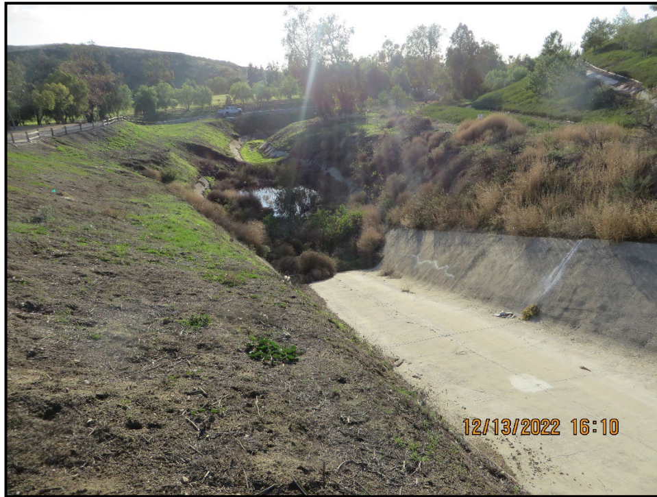
Photo 9) Spillway stilling basin looking downstream. Note trees and vegetation.
