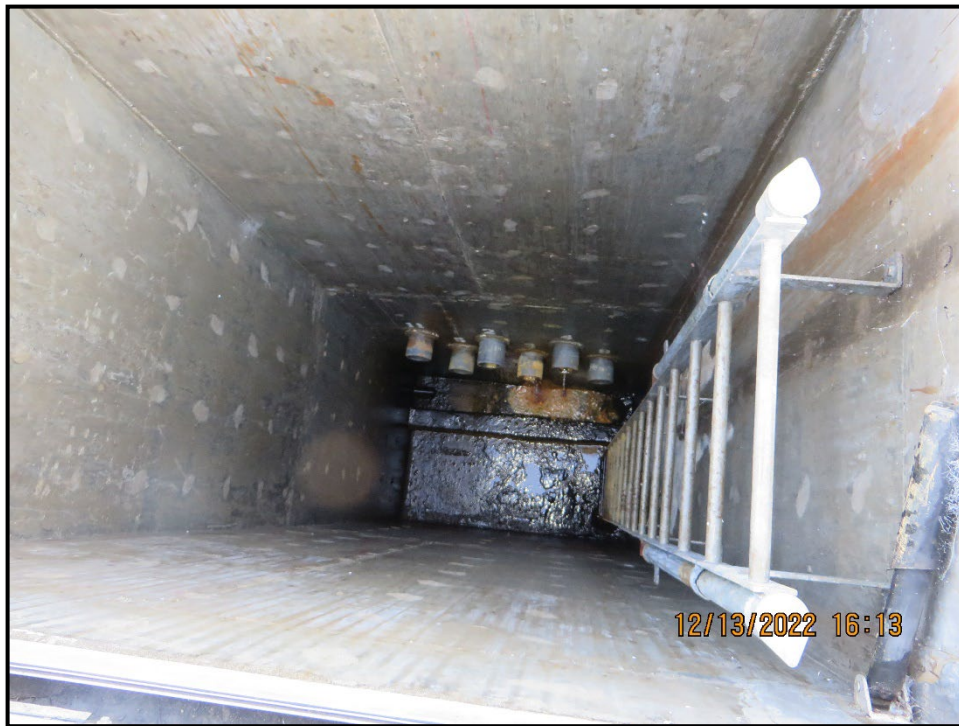
Photo 12) Seepage drain-pipe outfalls at the bottom of the seepage vault downstream of dam.
