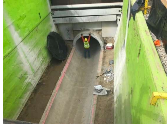
Rincon provided CEQA support, technical reports, and construction monitoring for rehabilitation of 100 miles of Prestressed Concrete Cylinder Pipelines for The Metropolitan Water District of Southern California
