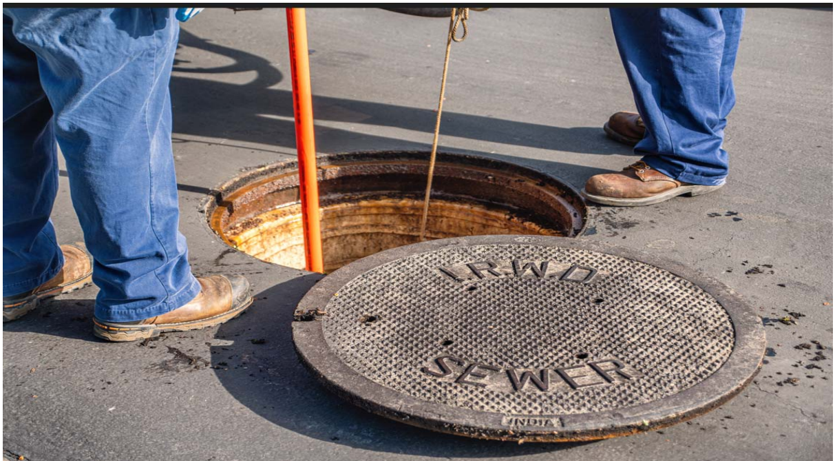
IRWD Manhole Cover
