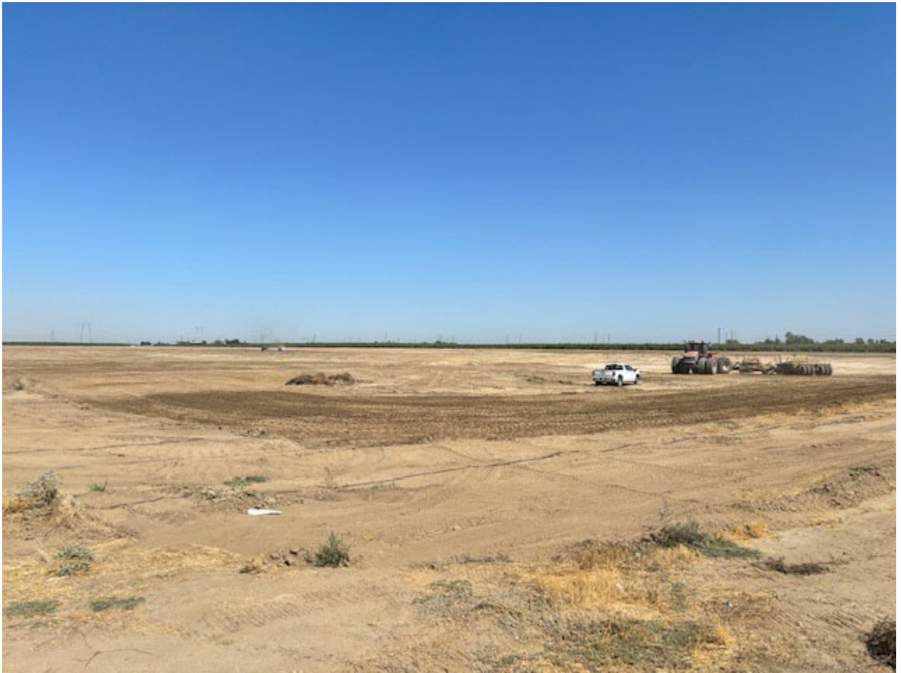
Backfill and Compaction for Levee Embankment around Well Site back to Original Grade
