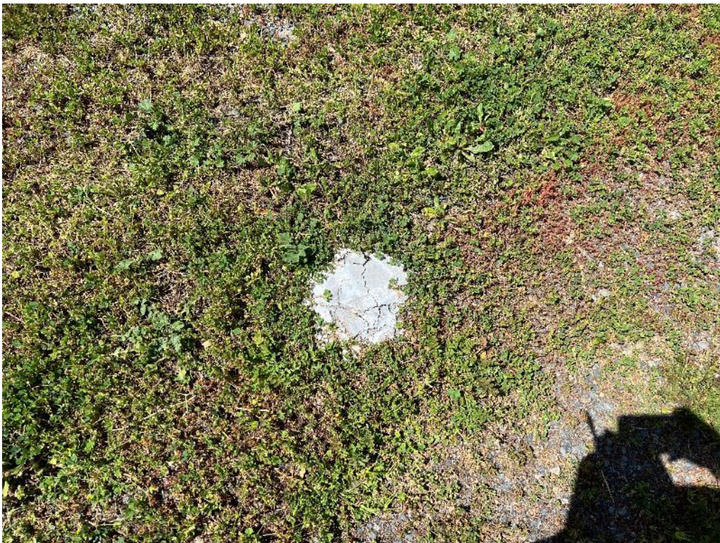
Photo 6. Example of boring in the downstream face of the embankment.
